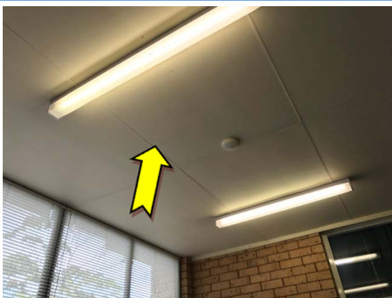
Photo 11. Interior, throughout, ceiling – suspected lead-containing cream upper paint system.
