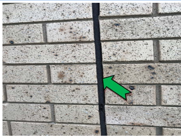
Photo 6. Exterior, throughout, wall joints – non asbestos-containing mastic sealant.
