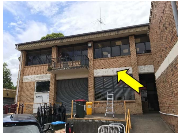
Photo 10. Exterior, north and south elevation, mid-level walls – suspected lead-containing beige upper paint system.
