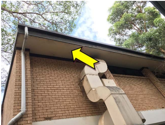
Photo 9. Exterior, north and south elevation, eaves – suspected lead-containing beige upper paint system.
